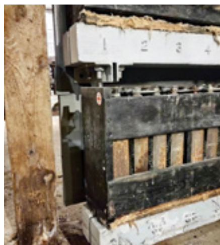
Part of the damaged structure and museum artefacts after the flooding at the Herring Era Museum.
