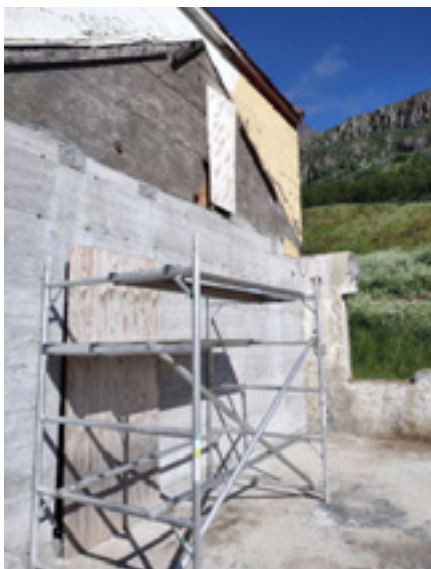
The new entrance to the Technical Museum of East Iceland, under construction during our visit in 2022. You can see where the landslide tore part of the building away.
